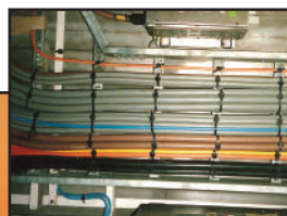
Marine Cable Bundling
