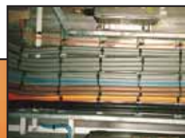
Marine Cable Bundling
